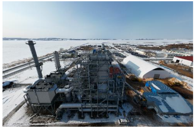
(3rd power plant)
