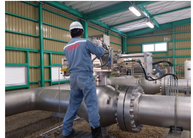
The Iwanuma Valve Station connecting with the Soma-Iwanuma Gas Pipeline
