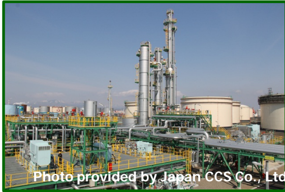
Ground facilities of CCS demonstration project in Tomakomai
