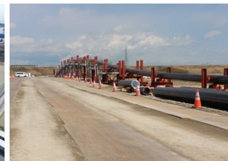
■ Connecting gas P/L between Soma and Iwanuma Installation work for arcuate long tube over the Abukuma river
