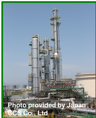
Facilities of CCS demonstration project in Tomakomai city
