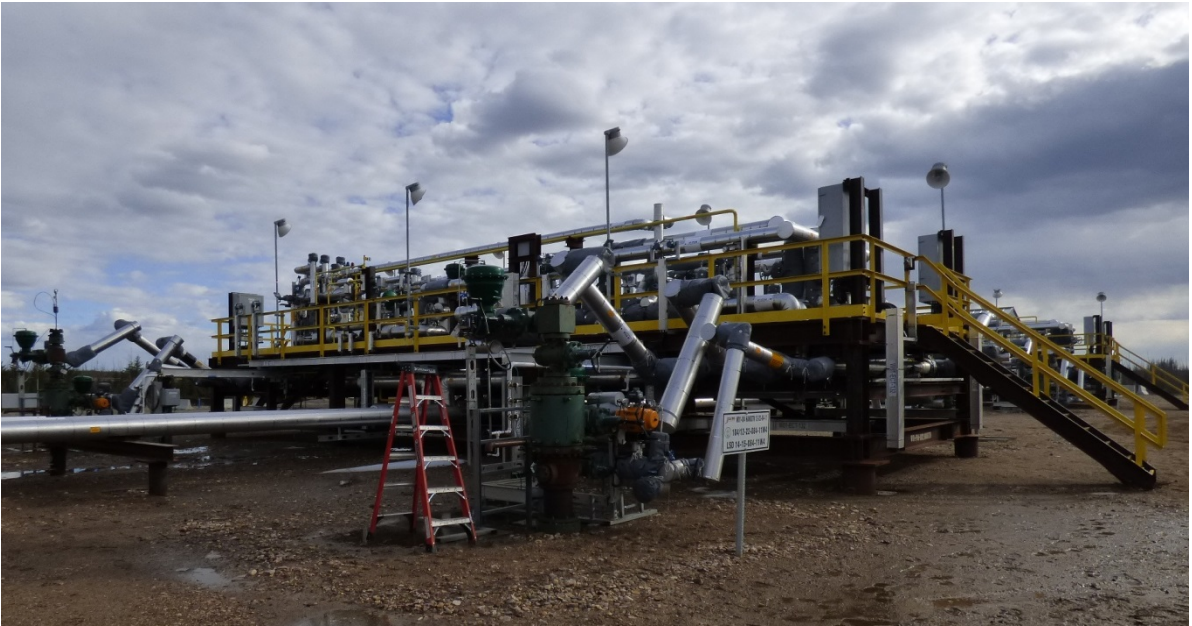
(Picture 2: Steam is being injected through the Wellhead facilities)
