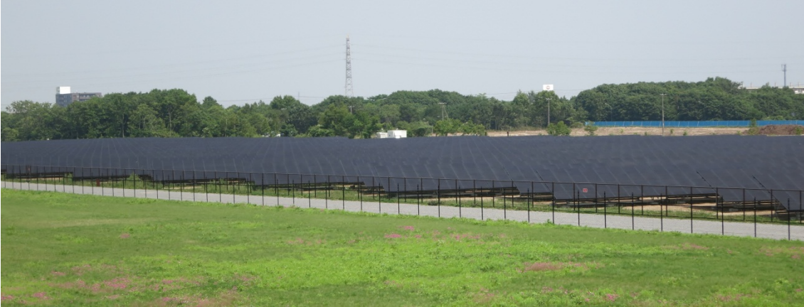
【Appearance of the mega-solar power station】
