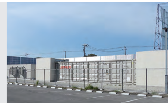
JAPEX Mihama Battery Energy Storage System
