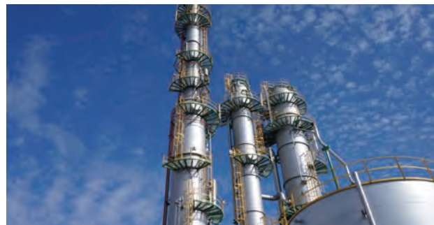
Aboveground facilities for demonstration project in Tomakomai (Photograph provided by Japan CCS Co., Ltd.)
