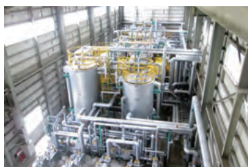
Crude oil processing facility of the Yufutsu Plant
