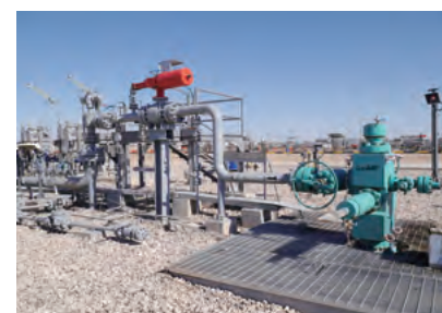
Garraf Oil Field production equipment
