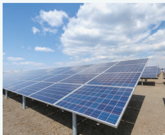
Solar panels (Solar Power Tomakomai Co., Ltd.)
