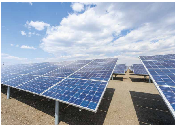
△ Our mega-solar power plant in Hokkaido
