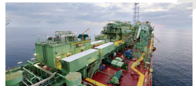
△ Offshore production facility
