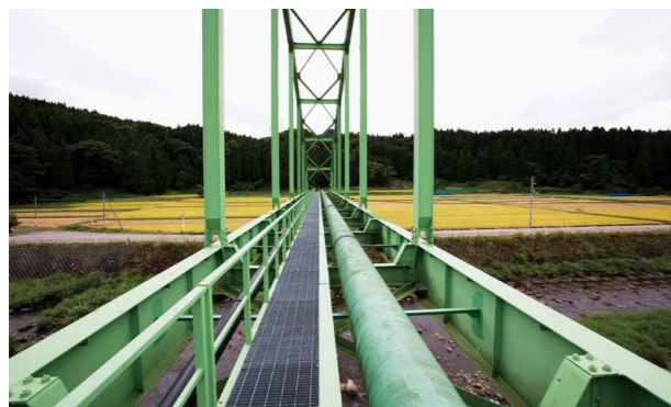
△ Niigata-Sendai Gas Pipeline
